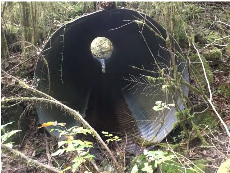
Inlet of overflowing of culvert
